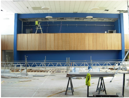
View from stage back to the Technical Gallery. New solid oak floor to be laid
