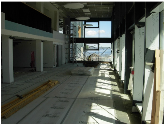
Ground floor café area, with views out to the Clyde and the Castle Gardens
