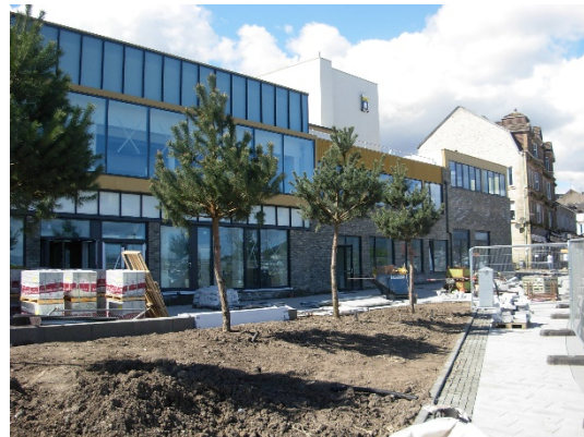
Eastern elevation – new glazed curtain walls, brickwork, cladding and public realm improvements (awaiting turf)
