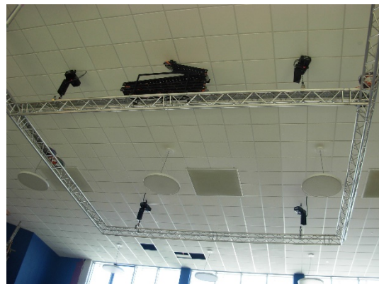
New ceiling, general lighting and fresh air vents. New figure-of-eight lighting rig suspended from 6 electric winches for ease of operation/maintenance.
