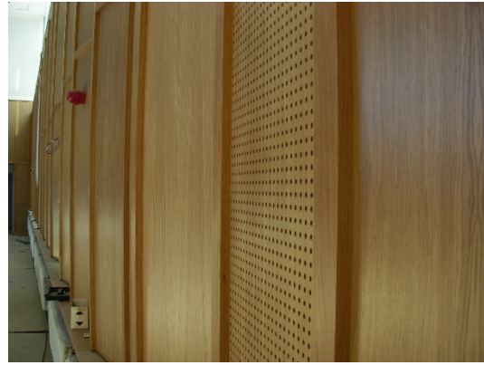
Acoustic wall panelling (absorption and reflection)
